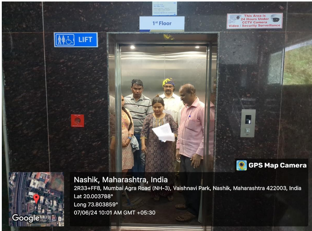
Lift in MDS Building
