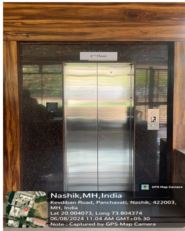
Lift in Principal Office Building
